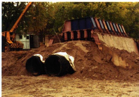
Vertical pressure is applied to the buried pipes in increments by applying pressure from the hydraulic jacks mounted on beams above the soil cover.
