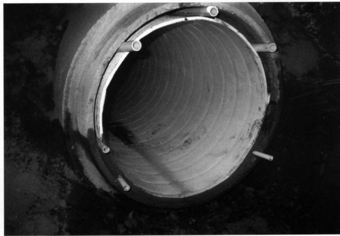
Filling and venting tubes are placed in the annular space around the pipe liner and a cement based bulkhead is formed around the circumference of the pipe between the liner and the host pipe.
