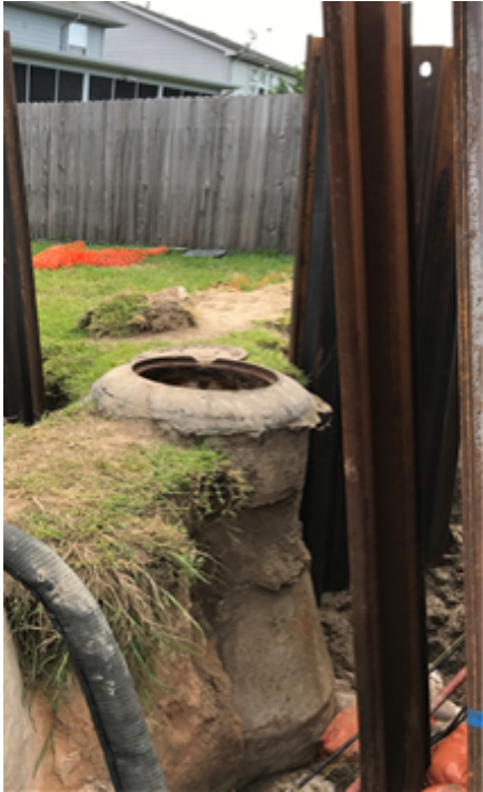
Floodwaters eroded soil
