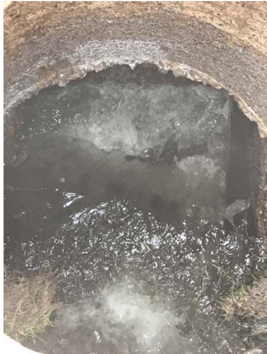
Breach in bottom of manhole
